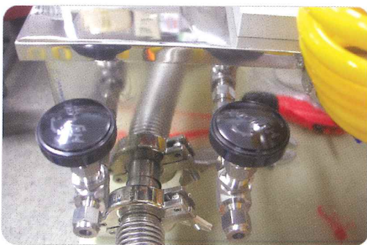
Gas valve to flow in and out chamber
